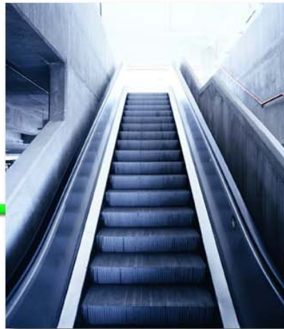
Escalator Shutdown ( 240V AC 5A )
