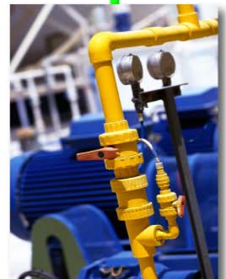
Valve Shutdown (30V DC 1A)
